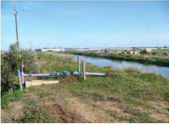
Figure 17.5. Recycled wastewater from the City of Adelaide, Australia, is pumped into an irrigation pond for a vegetable farm. Wastewater-conveying pipes are painted purple to distinguish them from freshwater conduits.
