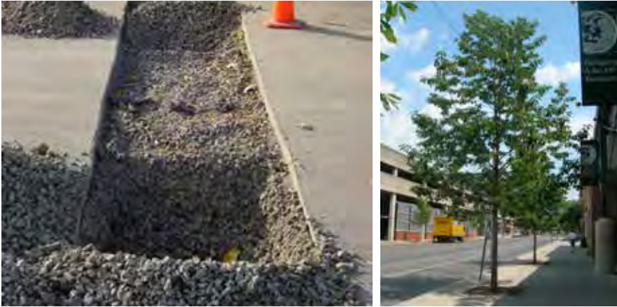
Figure 22.6. Left: Planting hole in gap-graded soil material that supports high loads from the pavement while allowing large pores for tree root protrusion. Pores are partially filled with fine soil particles and organic matter to provide plant growth functions. Right: Healthy street trees in a sidewalk with gap-graded soil. Photos by Cornell University, Urban Horticulture Institute.
